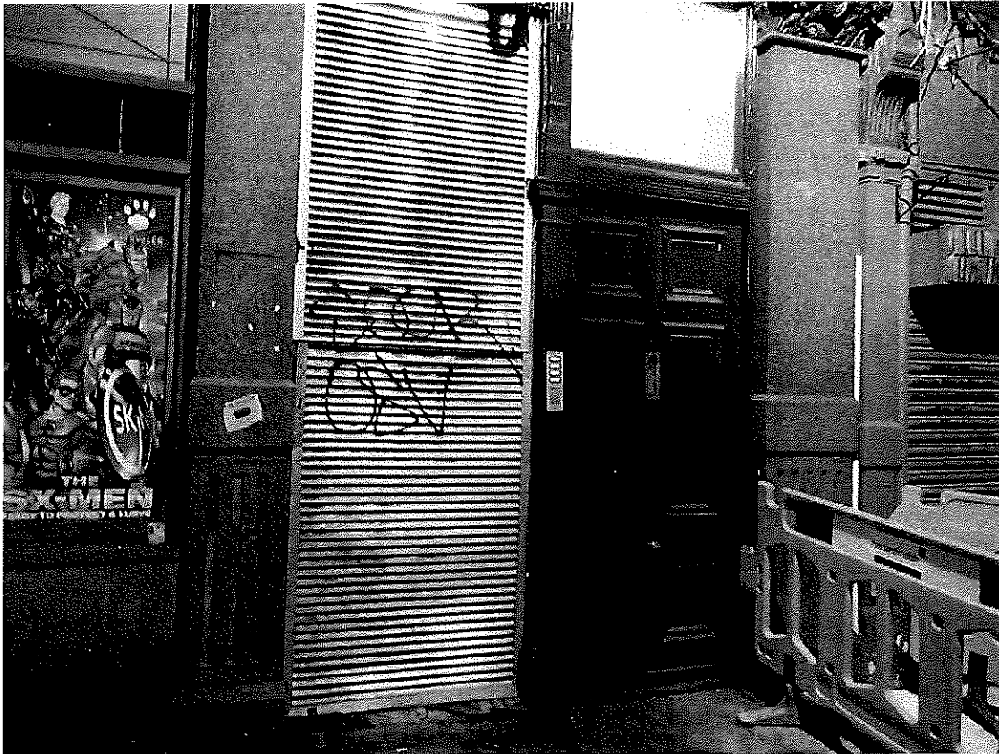
Figure 3: Mechanical plant louvres in Tisbury Court. The plant was operating through the night.
